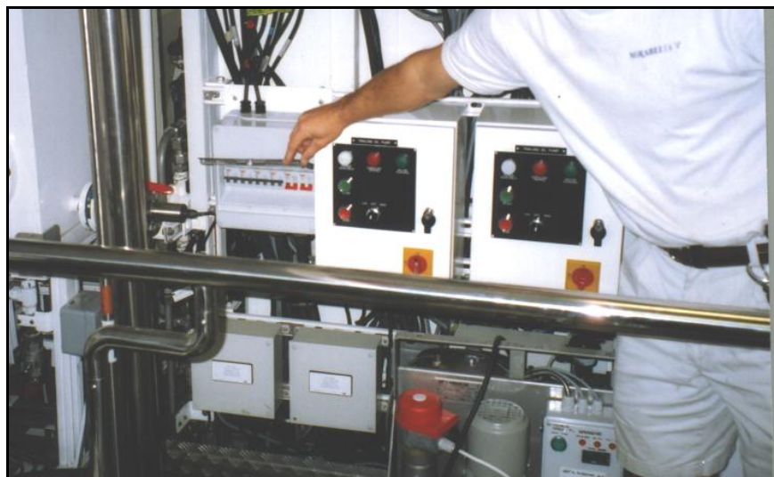
4. Main engine start electrical breakers
